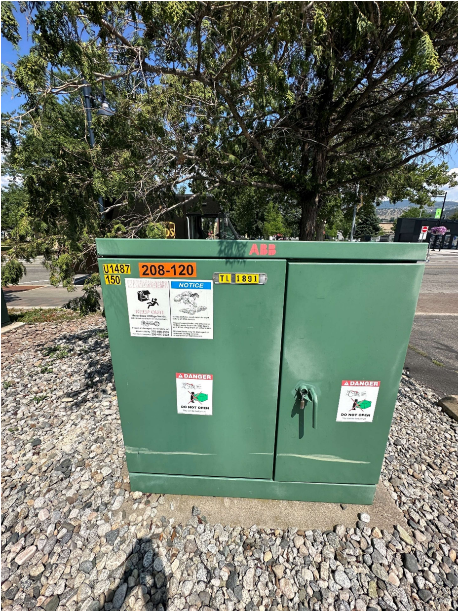
101 Martin Street – Existing 150 kVA Transformer
