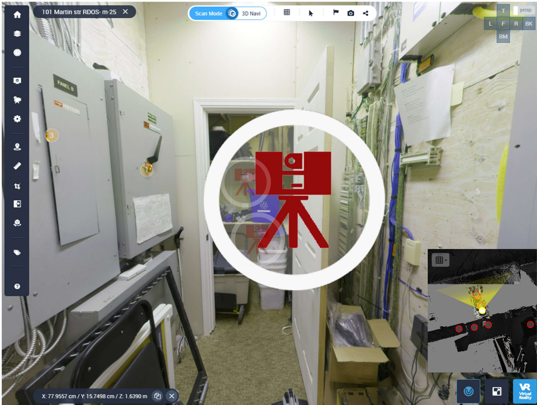
101 Martin Street Electrical Room
