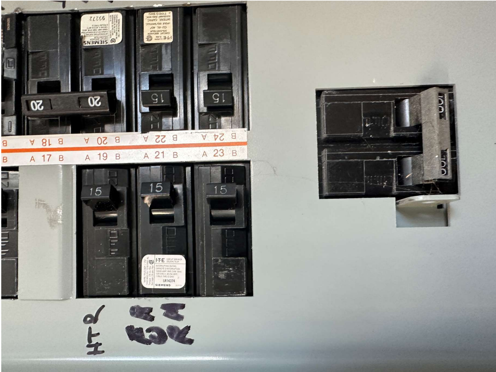
Willow Street – Main Panel
