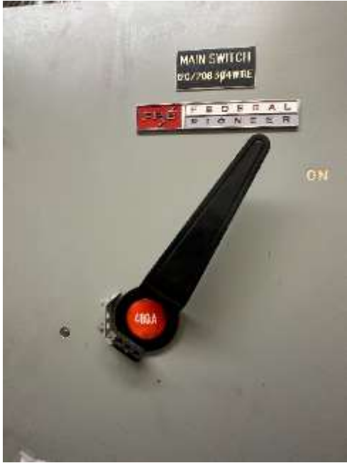
101 Martin Street Main Switch
