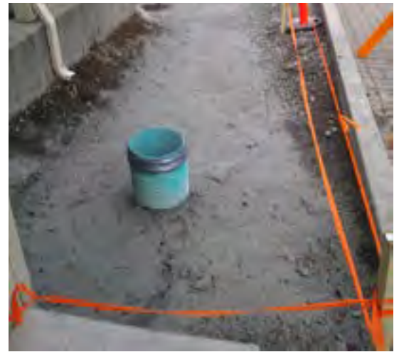
Image 4: Amending soil with clay barrier
