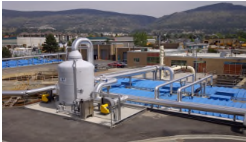
Photo 1: BIOREM biological removal system at the Penticton Wastewater Treatment Plant
