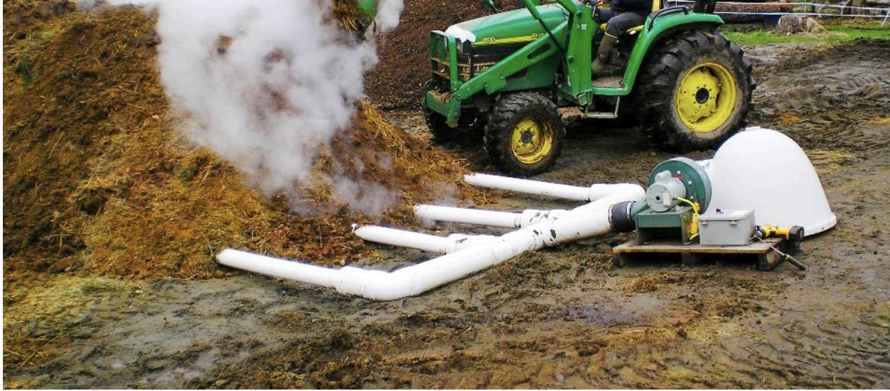
Figure 11. Example of forced aeration piping and blower system 24
