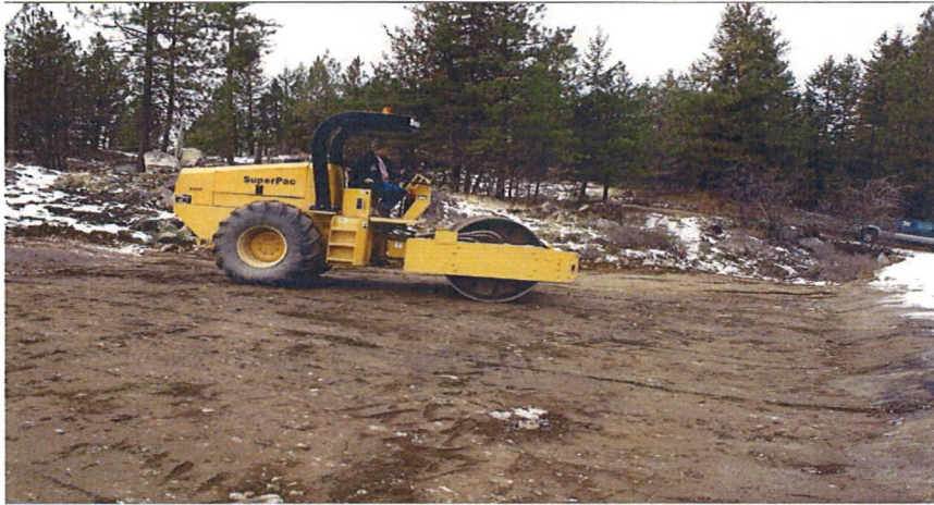
Building site preparation. Vegetation was cleared and burned to make way for services, landscape features and building sites. Fire Smarting. Frequently rock was blasted to level the building site.
