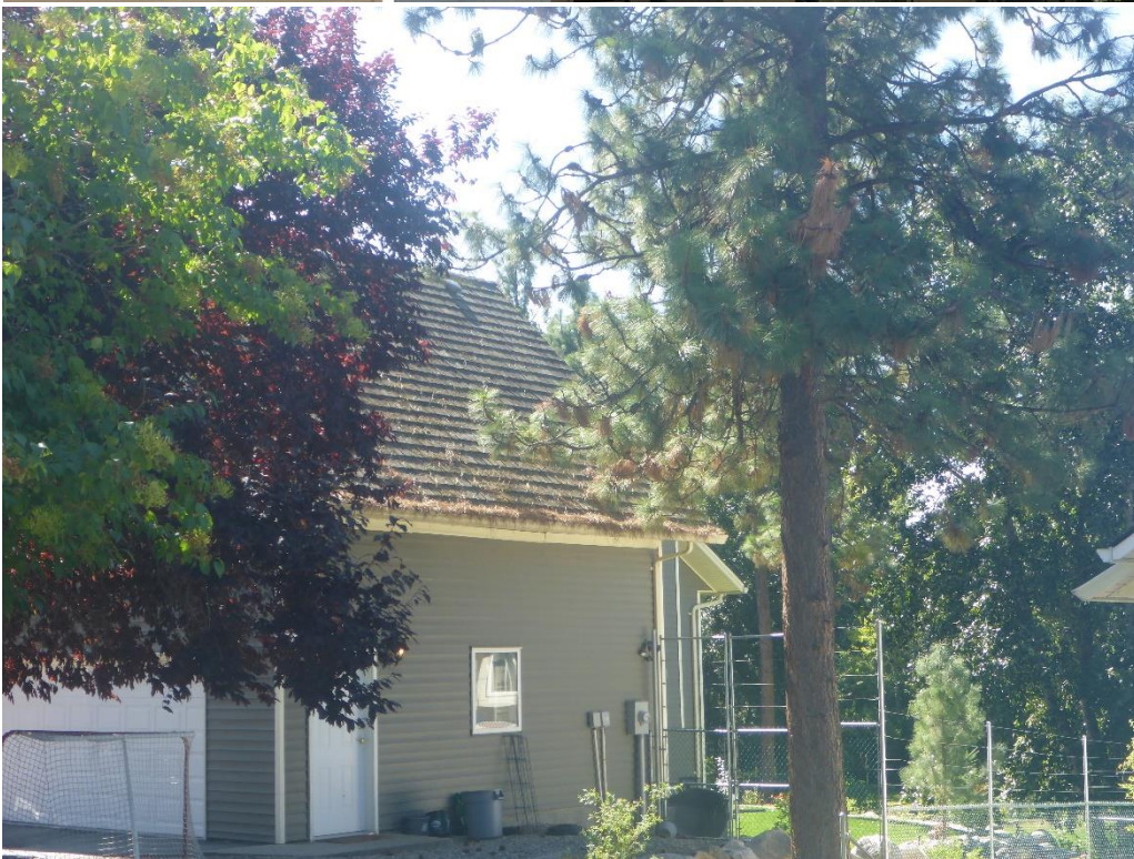
Figure 10. Non-compliant homes roofed in cedar shakes with accumulations of needles in gutters and crevices.
