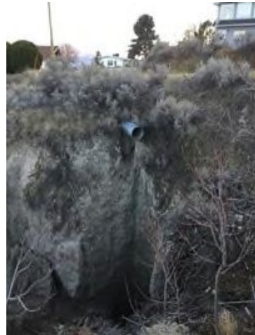
Photo 14 Massive sinkhole at culvert outlet (adj to Photo 13 Sage Mesa)
