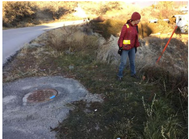
Photo 4 Catch basin above Sage Mesa Road at top of steep embankment (showing signs of instability)
