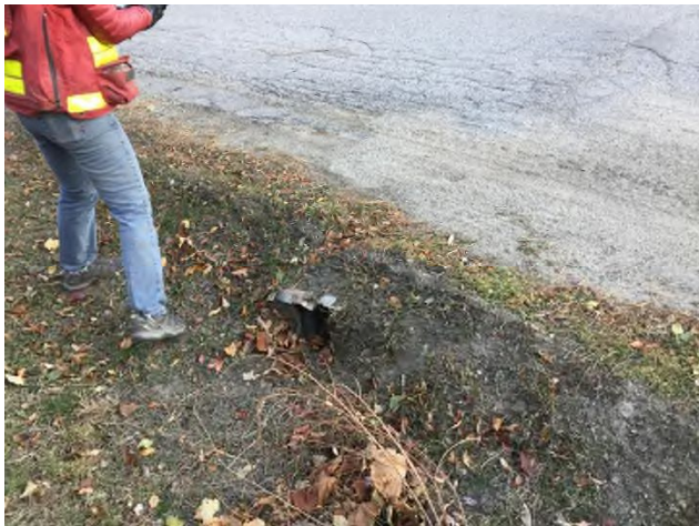
Photo 3 Damaged culvert inlet (Sage Mesa)
