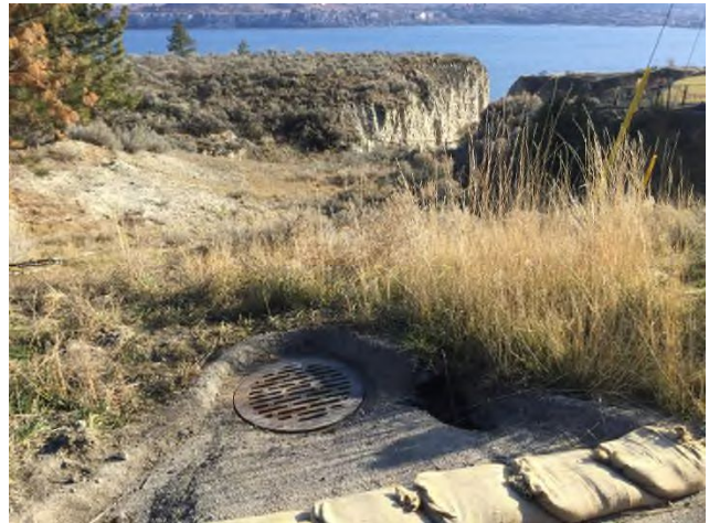
Photo 16 Sinkhole next to catch basin, with sandbags blocking runoff
