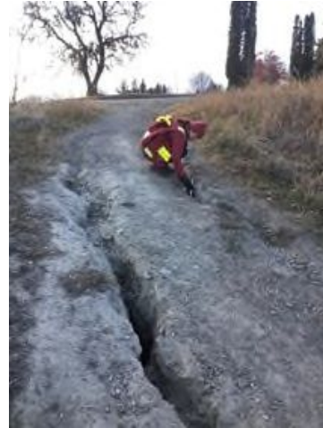
Photo 22 Subsurface erosion and deep cavity on access to KVR at Newton Road
