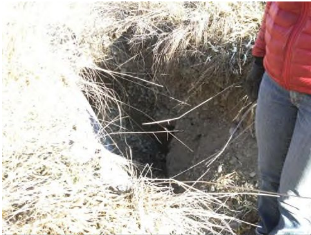
Photo 7 Erosion at Culvert Inlet at Sage Mesa Rd crossing (near WOW GC)
