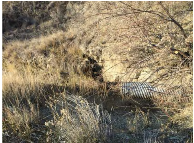
Photo 8 Erosion at culvert outlet at Sage Mesa Rd crossing (near WOW GC)
