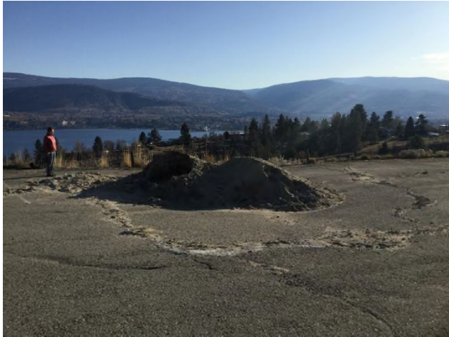
Photo 9 Large sinkhole forming in parking lot (WOW GC)
