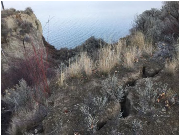
Photo 13 Tension crack at gully edge (Sage Mesa)
