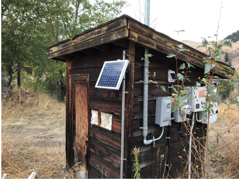
Photo 5 A view of the solar panel mounted on the shack.
