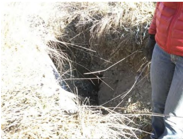
Photo 7 Erosion at Culvert Inlet at Sage Mesa Rd crossing (near WOW GC)
