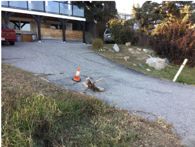
Photo 15 Small sinkhole in driveway (Sage Mesa)
