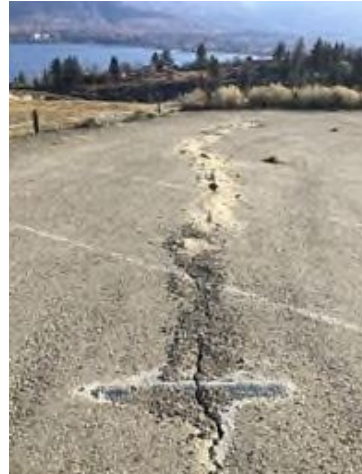
Photo 10 Pavement cracking at WOW GC
