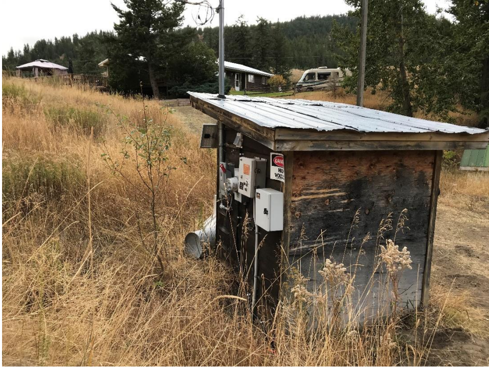
Photo 3 Utility control panel for LNID Pump and data logger, mounted on outside of shack located southeast of the pump.
