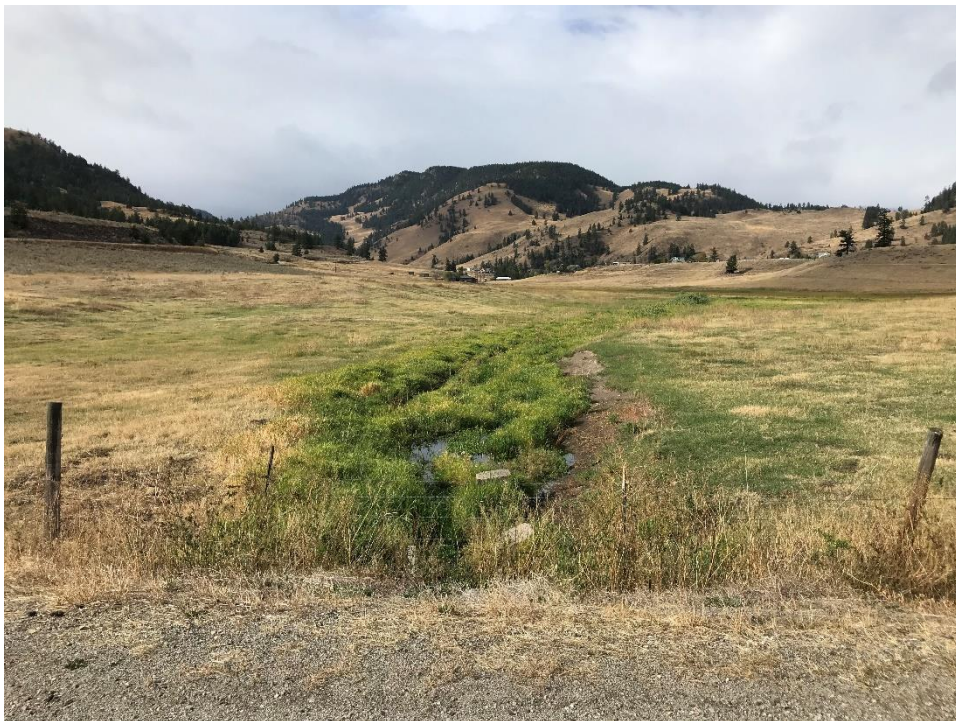
Photo 18 Standing over the culvert in Twin Lakes Road looking upstream at Lot 280.
