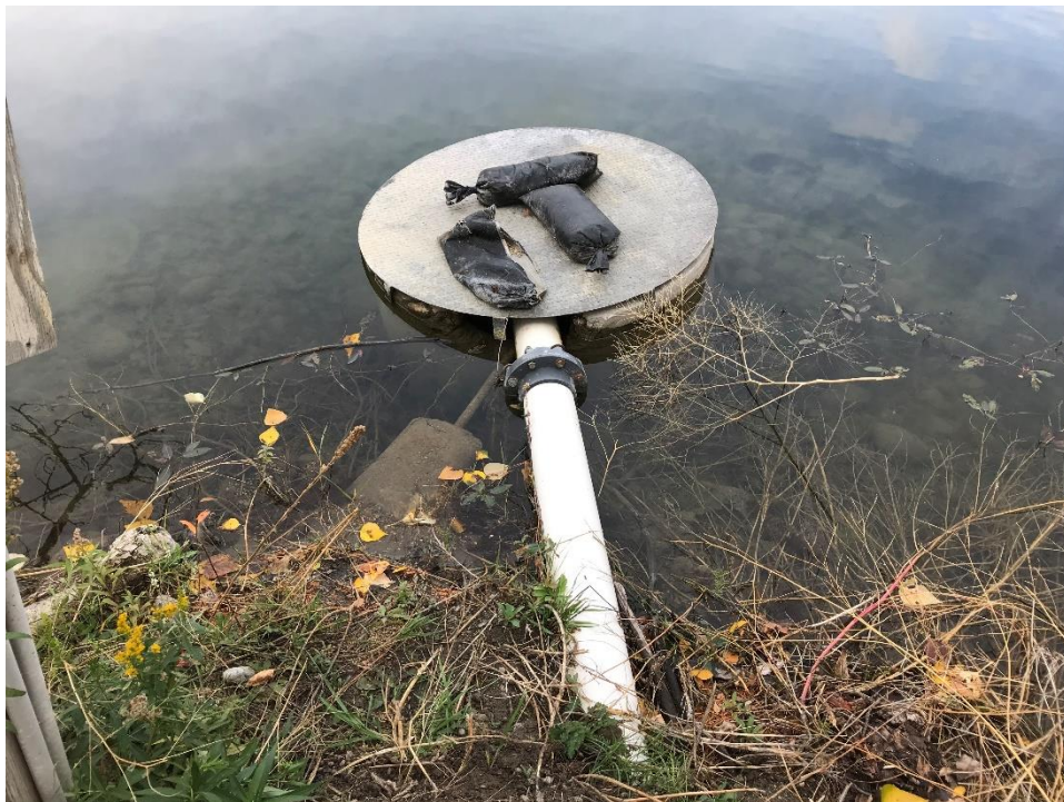
Photo 2 A closer look at the LNID pump, concrete housing and buried discharge piping.
