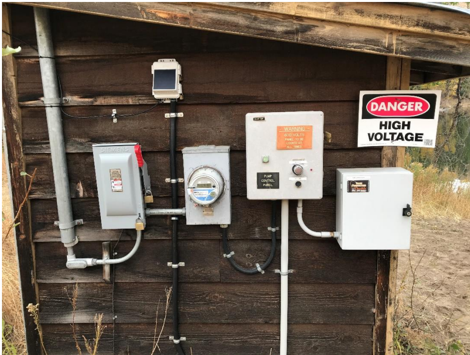
Photo 4 A closer look at the utility control panel for LNID Pump and data logger, mounted on outside of shack.
