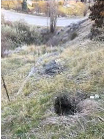
Photo 5 Sinkhole and tension crack near catch basin (see Photo 4)
