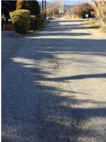
Photo 17 Depressions in road (end of Duchess Dr)
