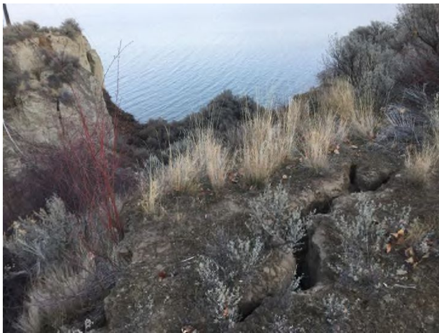
Photo 13 Tension crack at gully edge (Sage Mesa)
