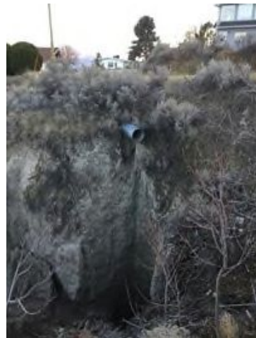
Photo 14 Massive sinkhole at culvert outlet (adj to Photo 13 Sage Mesa)
