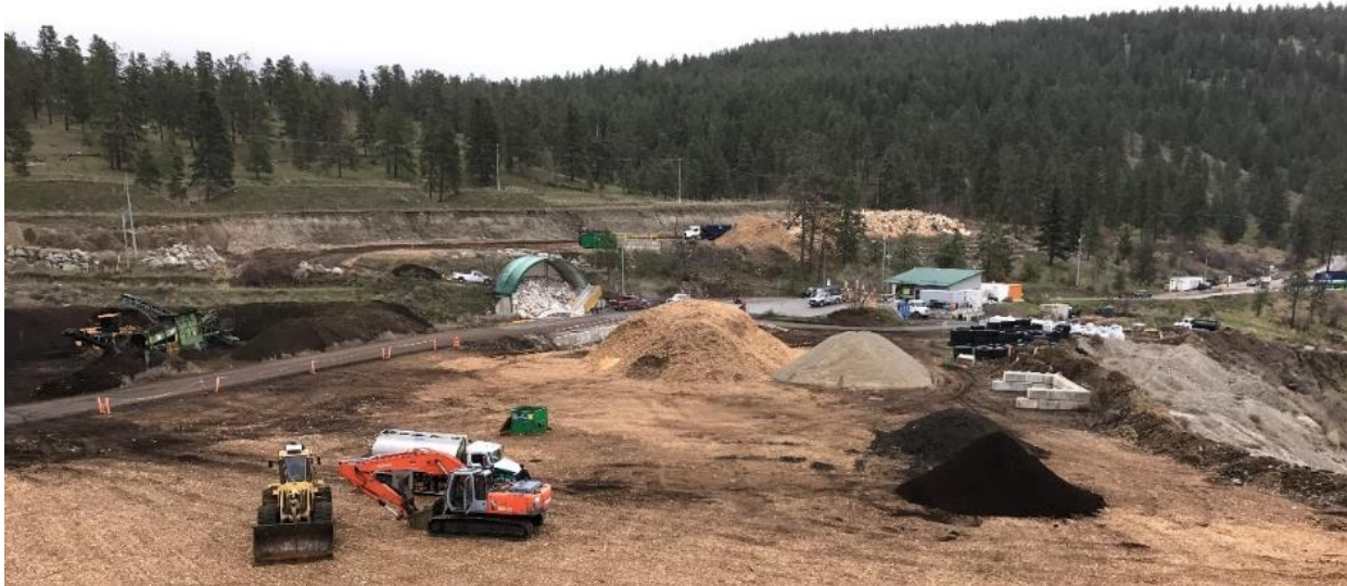
Photo 6 - The biocover blending area is shown in this photo. Note all feedstock material for the blending of the three (3) design mixes were sourced and delivered to site prior to blending.
