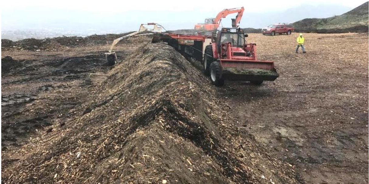
Photo 9 - 'Final-mix' being completed to the linear windrows with the 'Wildcat' Compost Turner.
