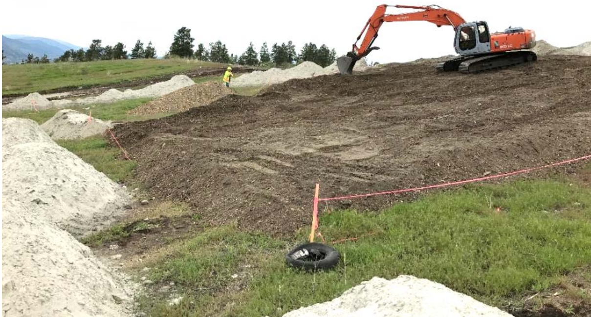
Photo 13 - The RDOS contractors spreading out biocover product in one mono lift ranging from 300-350mm in depth.
