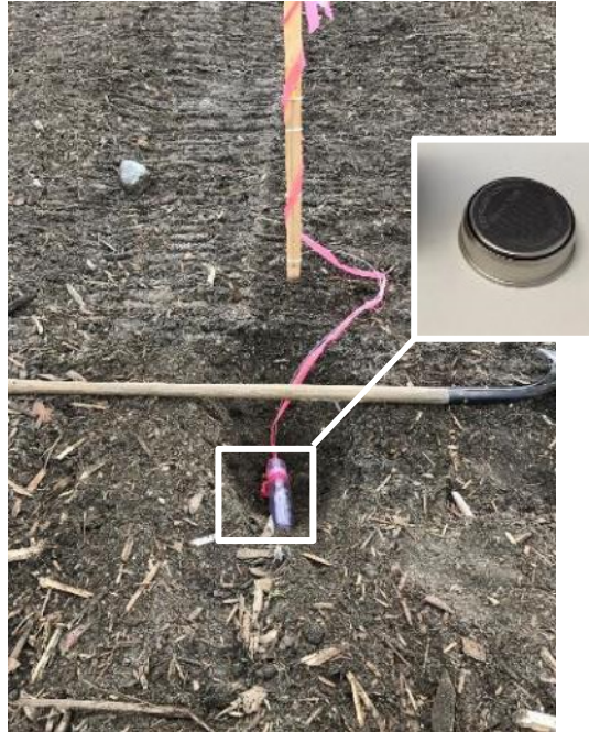
Photo 15 - Temperature probes (Smart Buttons), leashes and demarcation stakes installed in the biocover test pads.
