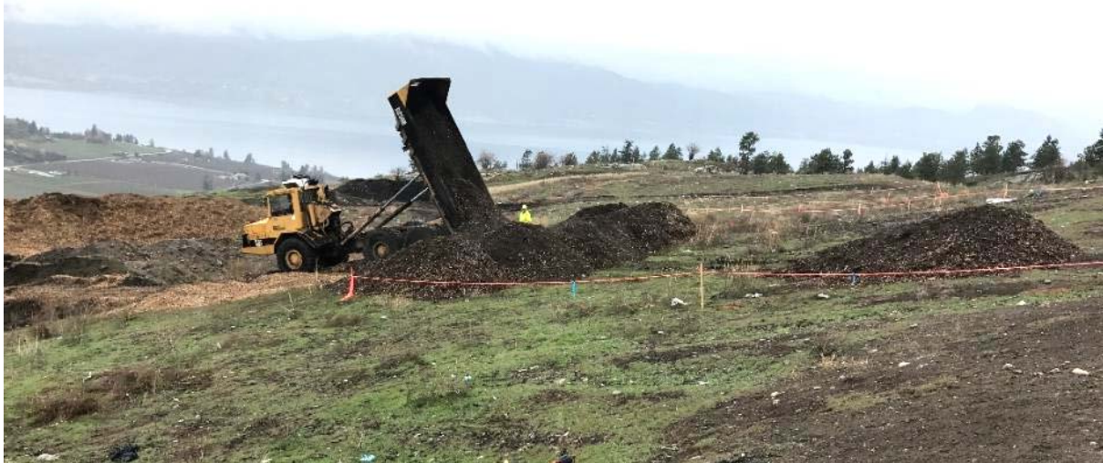
Photo 12 - Biocover product being hauled and stockpiled at each designated test pad site for construction.
