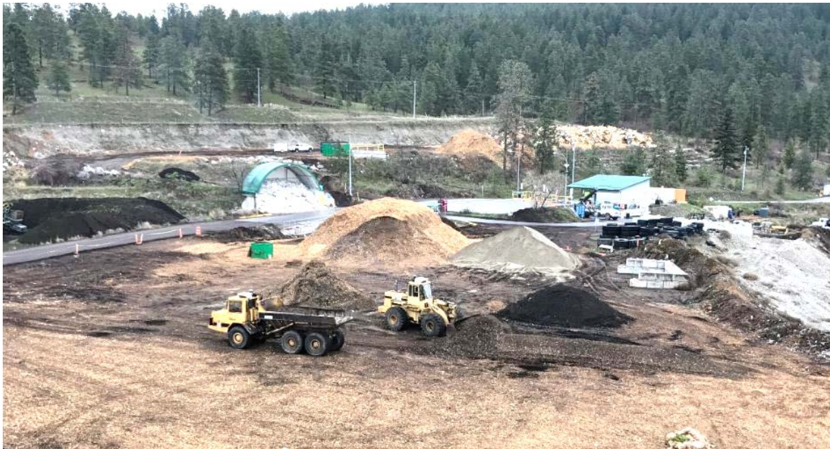
Photo 11 - Blended biocover material being loaded into off-road trucks from the blending site and hauled to the western slopes of the landfill.
