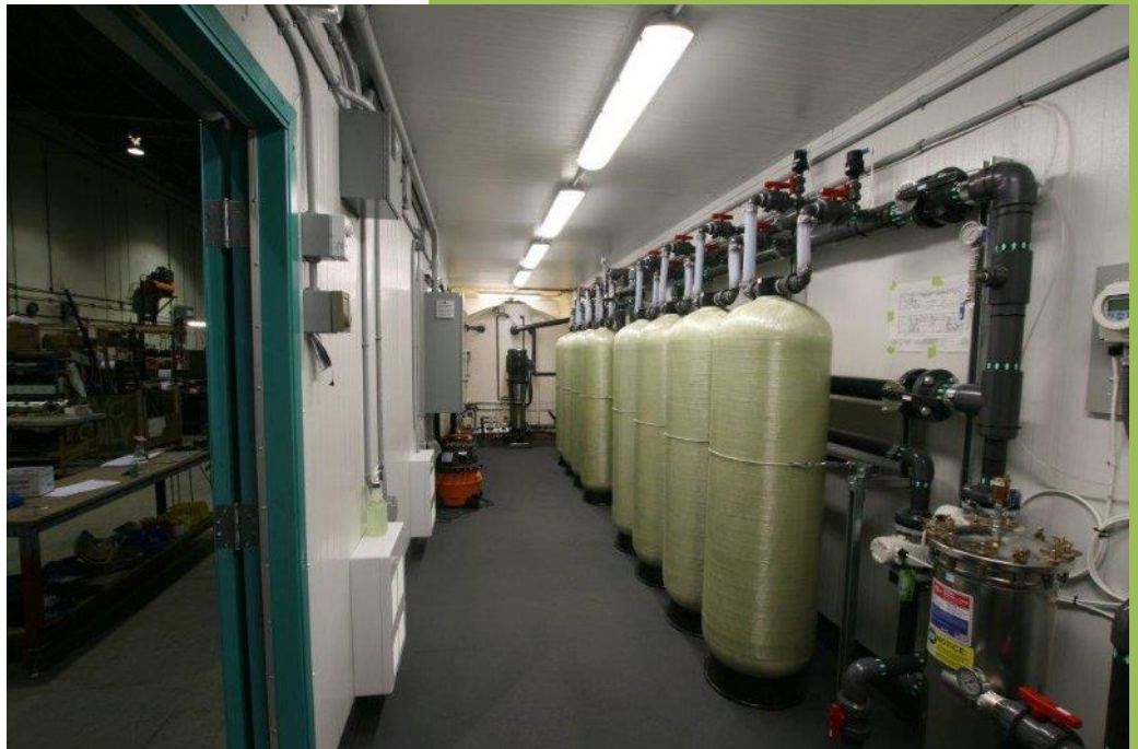
Faulder Uranium Treatment System
