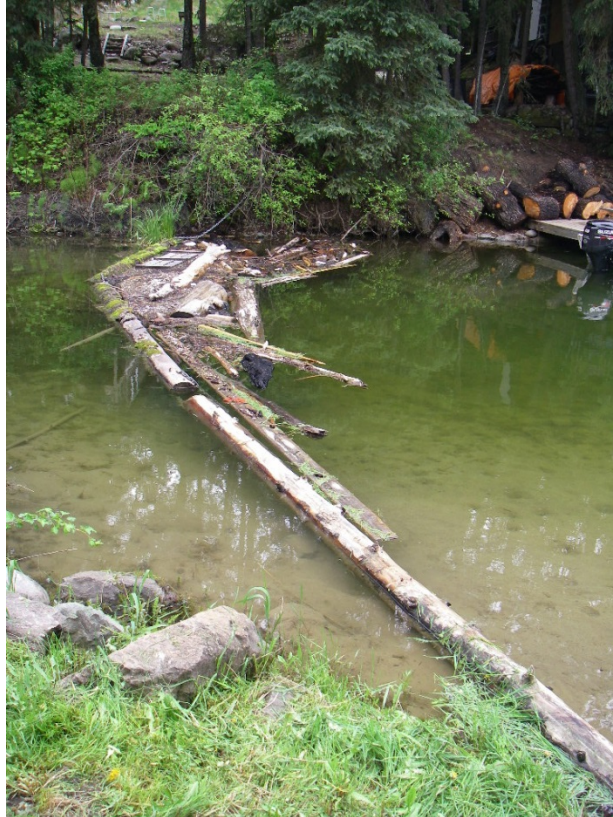
Debris at the log boom will be removed in the fall when water levels are lower.
