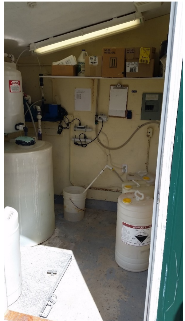
Inside of Chlorination Building – built in 2002
