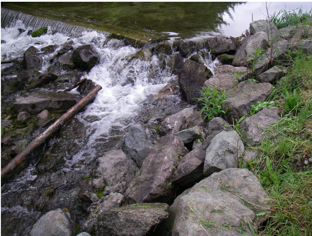
Rock rip rap along left bank downstream. Note voids between the individual rocks.
