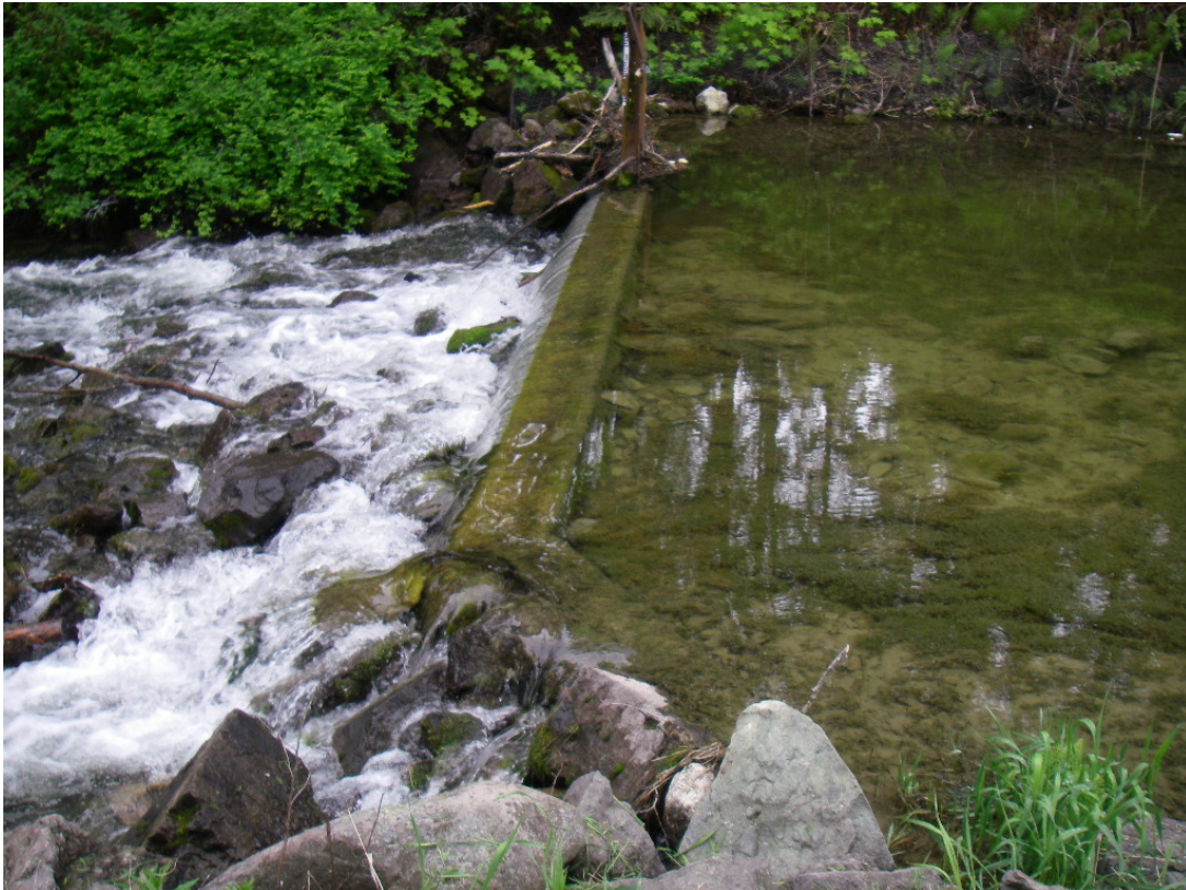
Looking across weir. Gate is at the far end. Debris around the gate was removed.
