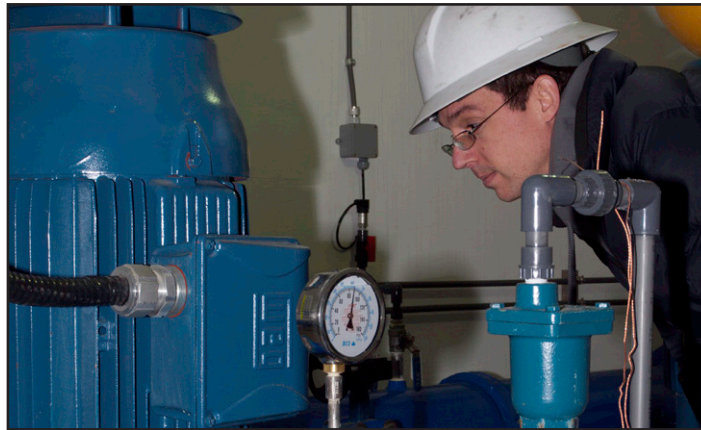
RDOS Environmental Technician Rob Palmer inside the West Bench booster station.
