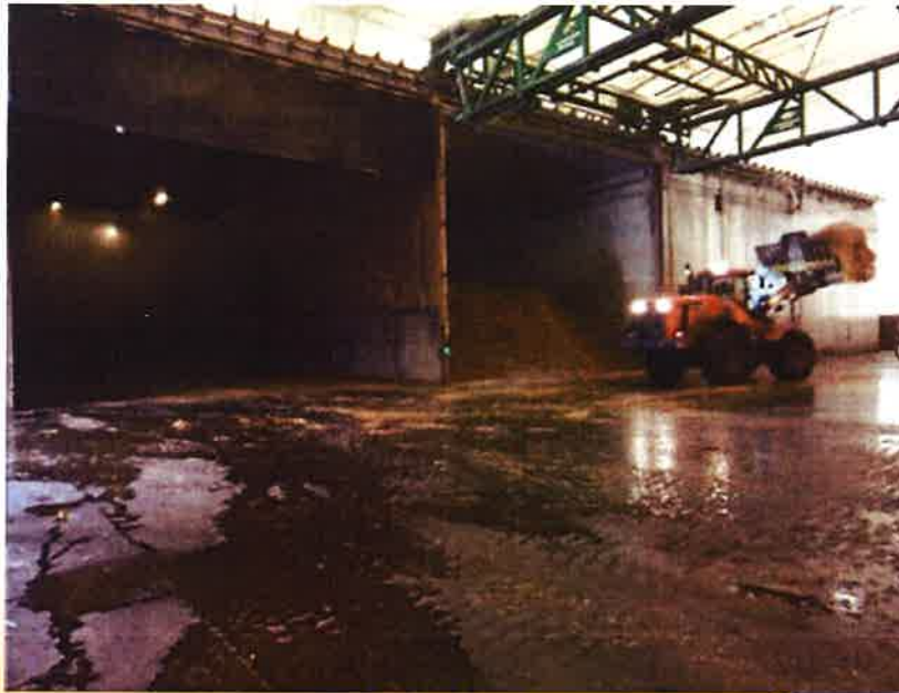
Enclosed Bunker System
