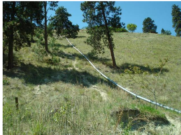
Photo 31: Drain pipe contains water across potentially unstable slopes north of Kaleden (Segment 15).
