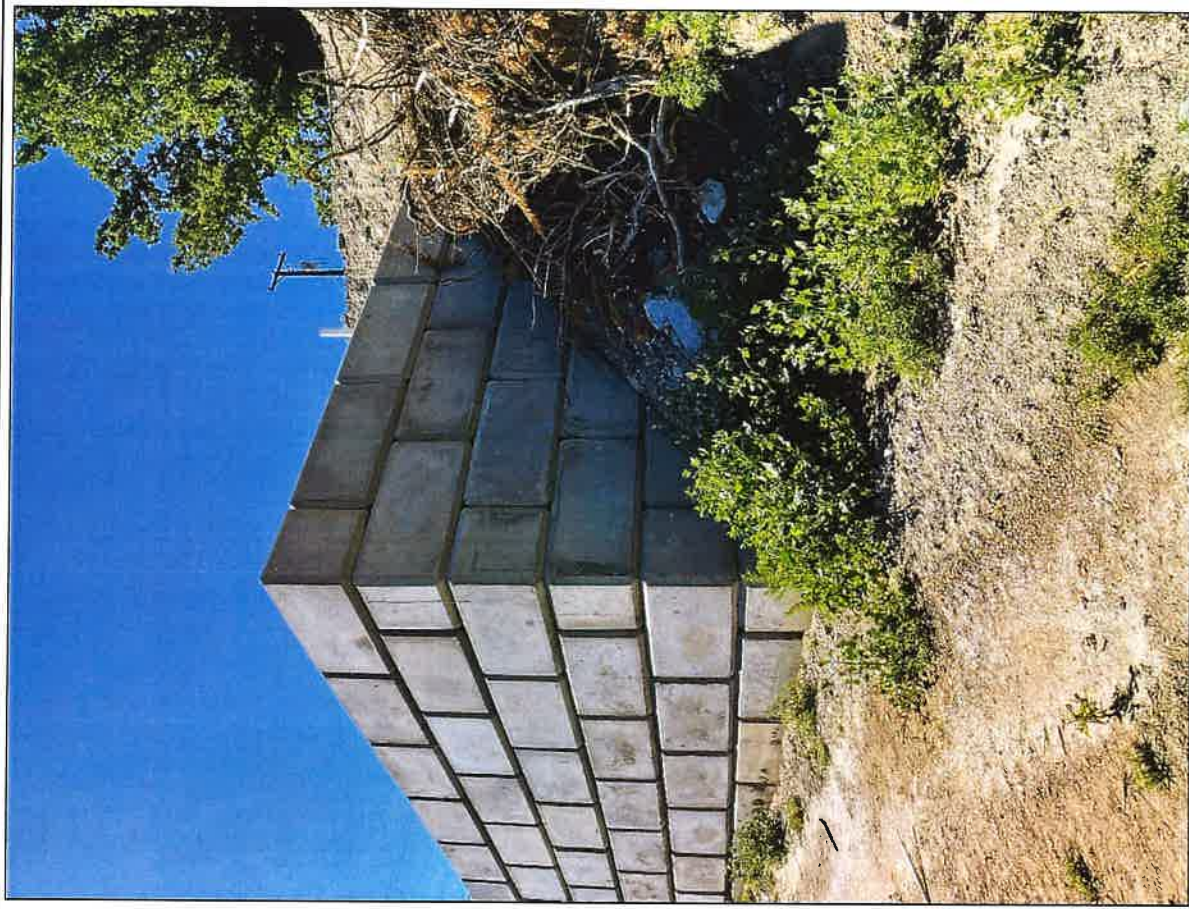
Image 2 - Highest point of retaining wall from subject parcel facing south towards Highway 97.
